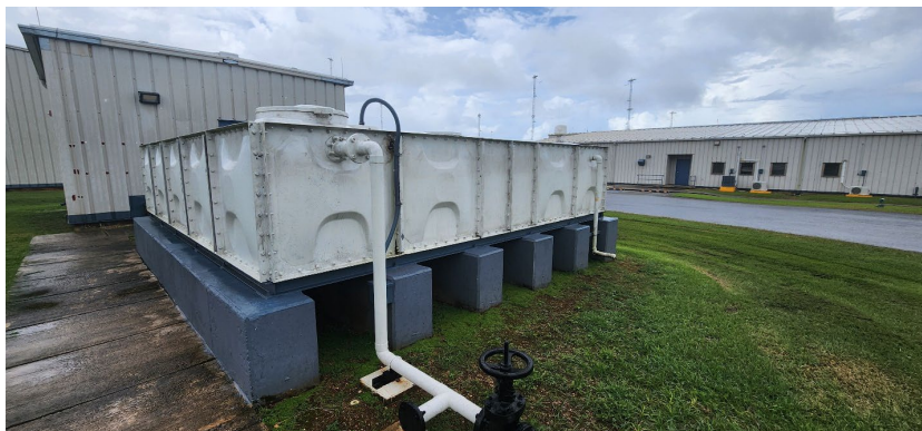
Figure 12 Non-potable Water Storage Tank at U.S. Agency for Global Media Facility on Tinian
