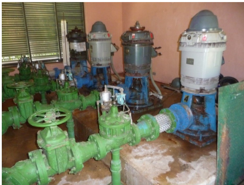
Figure 6 Maui Well No. 2 Pump Equipment
