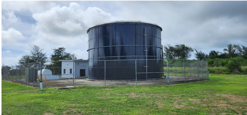
Figure 11 Water Tank and Booster Pump Station at Francisco Manglona Borja/Tinian International Airport
