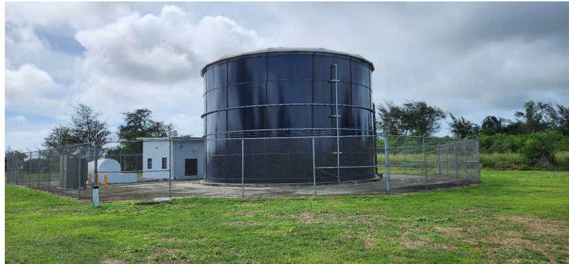
Figure 11 Water Tank and Booster Pump Station at Francisco Manglona Borja/Tinian International Airport
