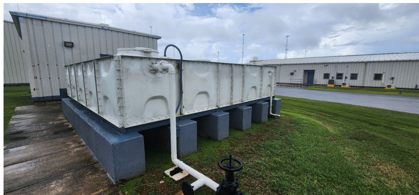
Figure 12 Non-potable Water Storage Tank at U.S. Agency for Global Media Facility on Tinian
